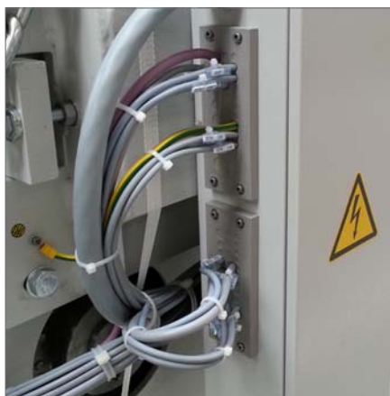
KEL-DPZ 24|x - Page 52 - 53 Routing of numerous cables with varying cable diameter sizes into a machine control panel. IP65 sealing is achieved. Additional membranes are available for future routing.
