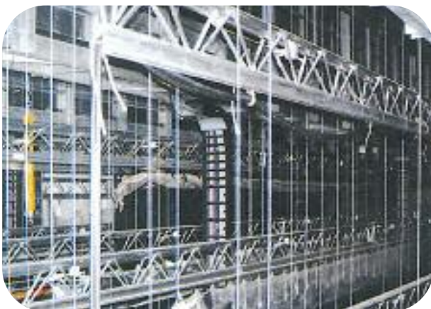
igus® ReadyChain® used for a zigzag application of an illumination cross arm, Royal Opera, London
